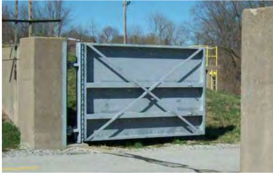
Figure 10: Swing Gate Closure Structure
