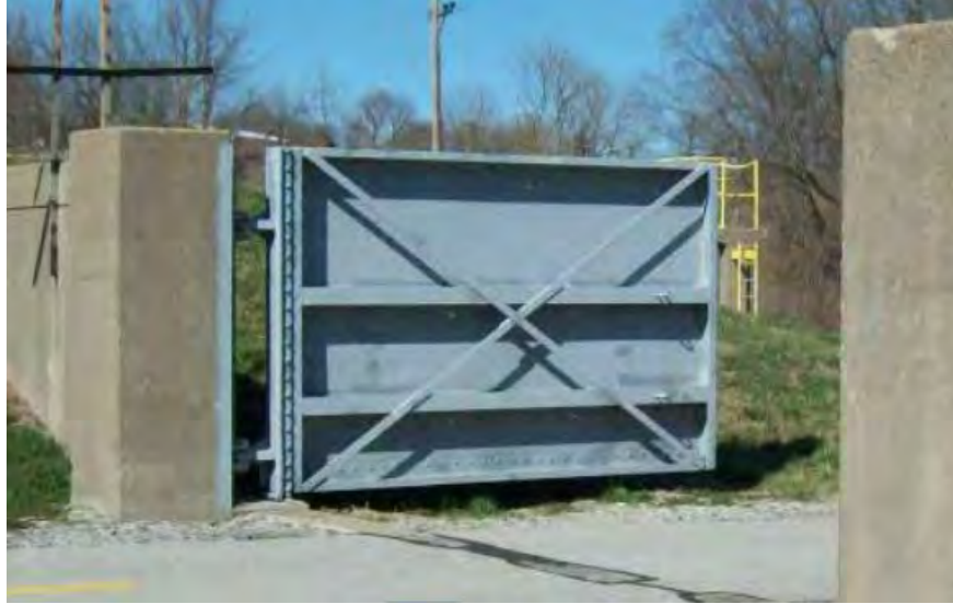
Figure 10: Swing Gate Closure Structure
