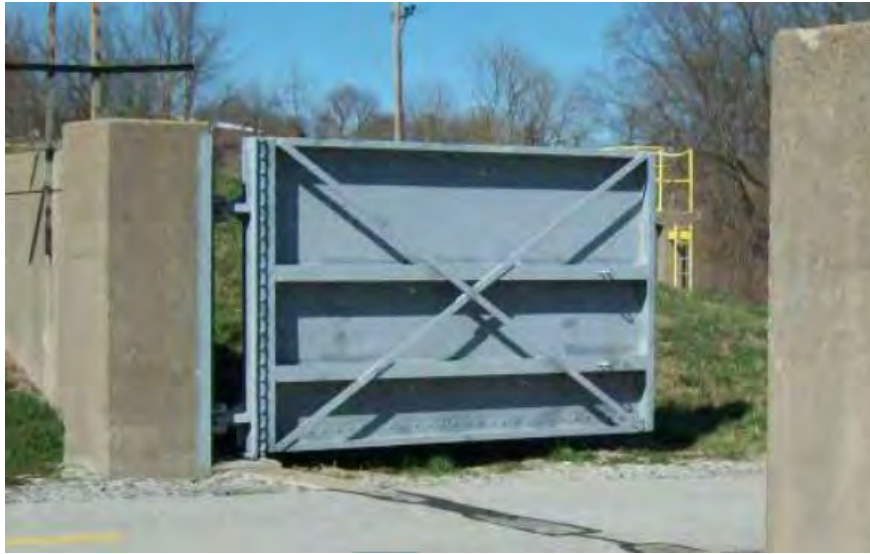
Figure 3: Swing Gate Closure Structure
