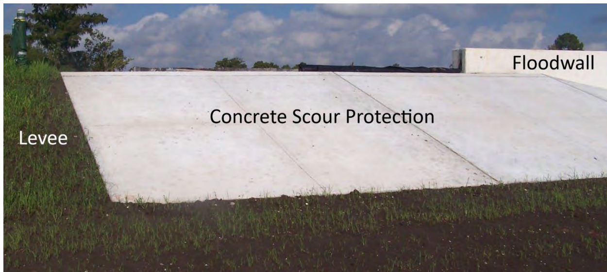
Figure 11: Concrete Scour Protection Example
