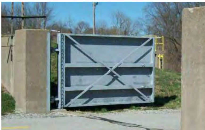
Figure 10: Swing Gate Closure Structure
