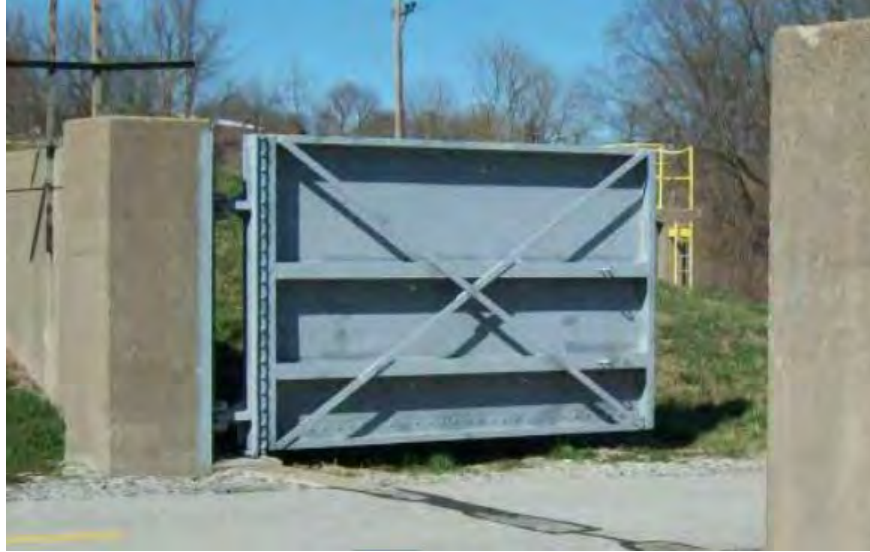
Figure 12: Swing Gate Closure Structure
